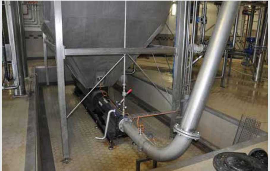
Seen here in the Victory Brewing Company Parkesburg facility, a patented auger feed at the base of the inlet hopper over-feeds the wet but non-flowing spent grain into the NETZSCH NEMO® progressing cavity pump (pump 1) to assure conveyance.
