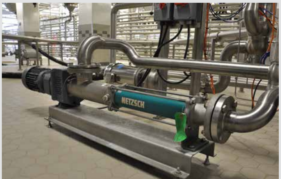
Over the course of brewing, the yeast involved in brewing can quadruple in quantity. This spent yeast is removed from the liquid through filtering, suctioning or settling. (pumps 4 & 5).
